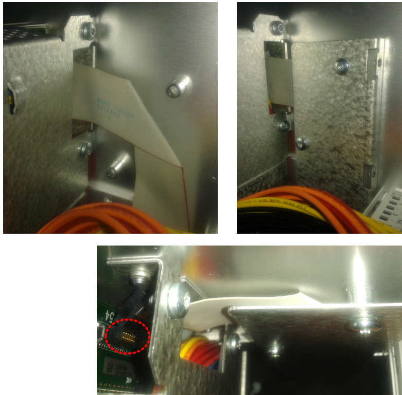
Fig. 3-8 Connecting the flat ribbon cable with the backplane. The counterplug is circled in red.
