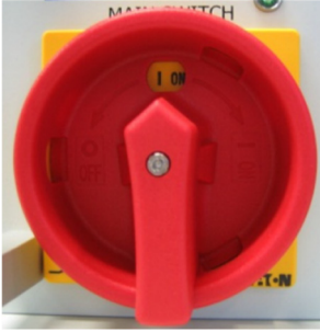
Ana şalter (MAIN SWITCH)
