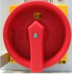
Ana şalter (MAIN SWITCH)
