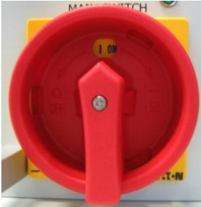
總開關 ( MAIN SWITCH )
